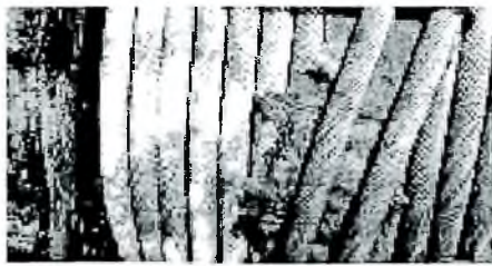
FIG. 1. CORROSION IN CONDUCTOR-A
