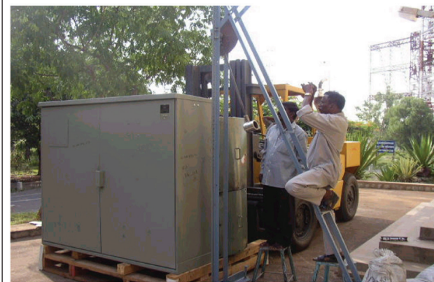
UNIT SUBSTATION ASSEMBLY (13.8 kV/231 kVA TRANSFORMER, HV COMPARTMENT AND LV PANEL CABIN AND ASSOCIATED HARDWARE) TESTED FOR M/S MOHAMMED AL-OJAIMI FACTORY, SAUDI ARABIA
