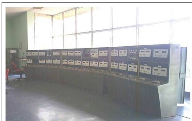
OLD CONTROL ROOM
