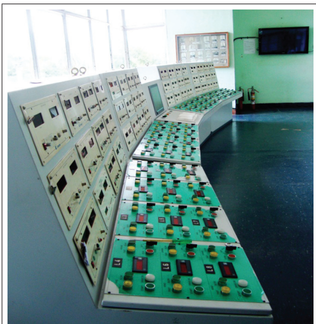
PLC CONTROL FACILITY, VIDEO FACILITY
