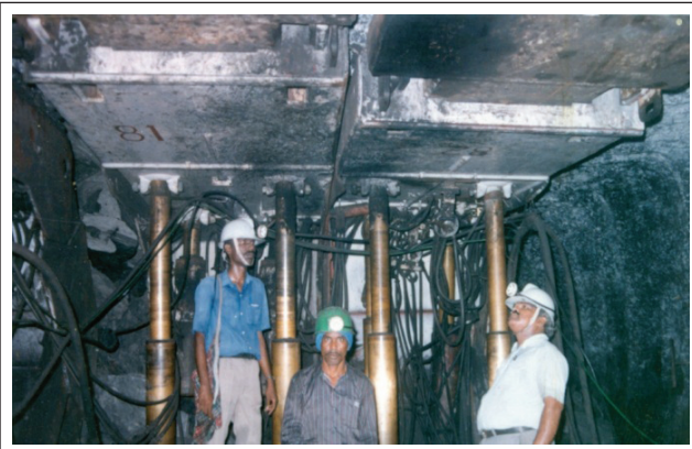
INSTALLATION AND COMMISSIONING OF PROJECT 'POWERED SUPPORT CHARACTERISTICS RECORDER' IN UNDERGROUND COAL MINE NEAR DHANBAD (BIHAR STATE)
