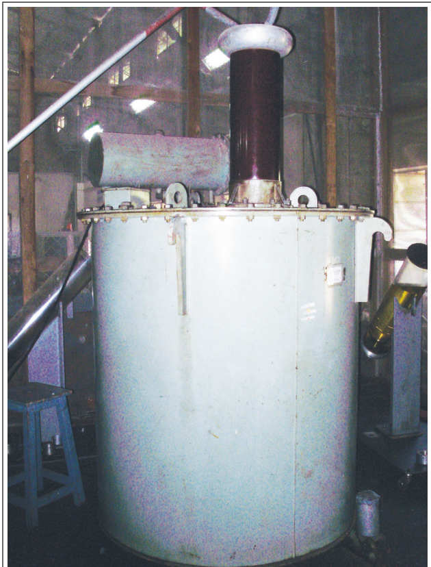
FIG. 2 100 kV AC, PD FREE TRANSFORMER
