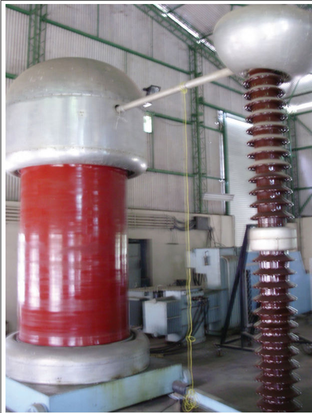
FIG. 10 300 kV AC TEST SOURCE WITH DIVIDER
