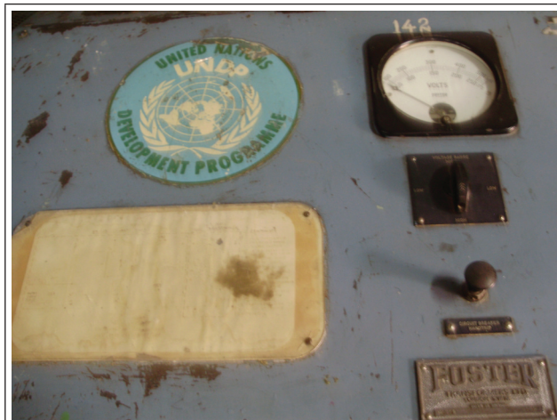
FIG. 4 A VIEW OF CONTROL PANEL
