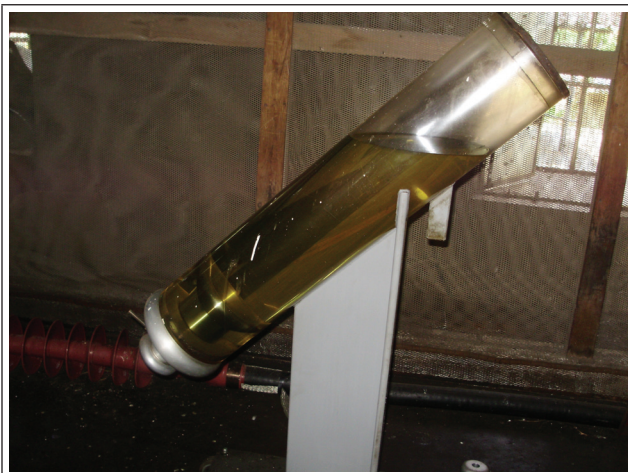
FIG. 7 A VIEW OF 66 kV CABLE TERMINATION
