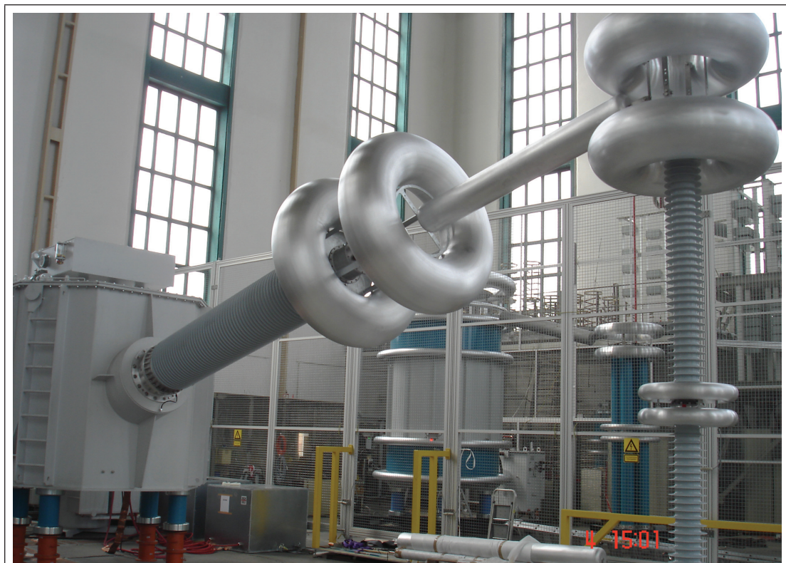
FIG. 26 A VIEW OF 600 kV, 4200 kVA AC TEST SYSTEM
