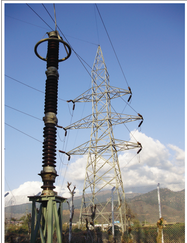
A VIEW OF LIGHTNING ARRESTER
