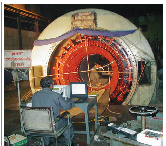
A VIEW OF ELCID TEST ON TERBO GENERATOR IN PROGRESS
