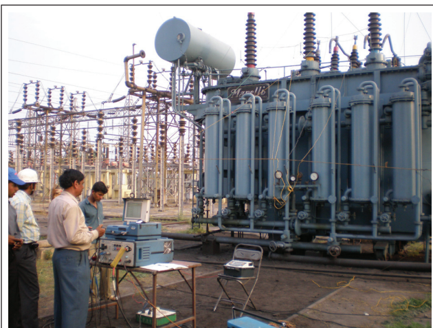
A VIEW OF TAN- \delta TEST ON TRANSFORMER IN PROGRESS
