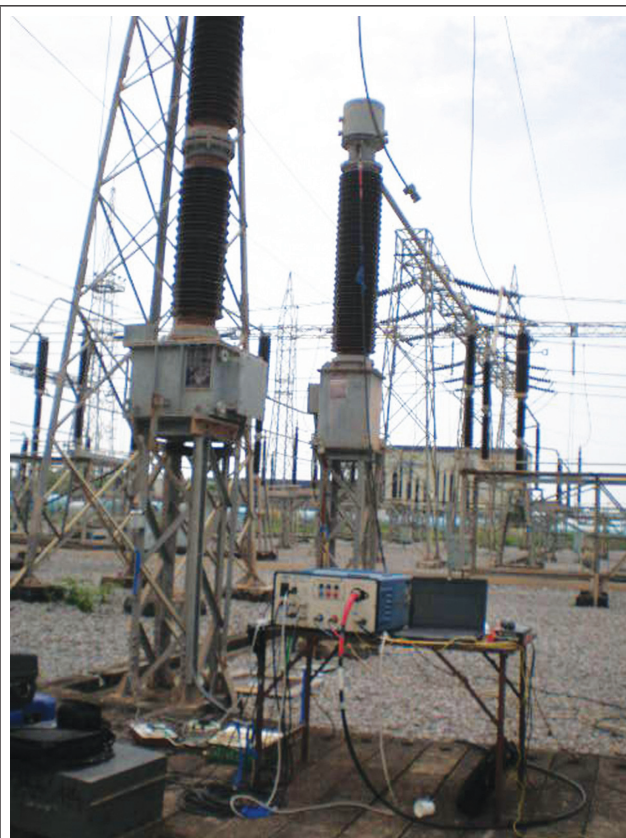
A VIEW OF TAN- \delta TEST ON CTs IN PROGRESS
