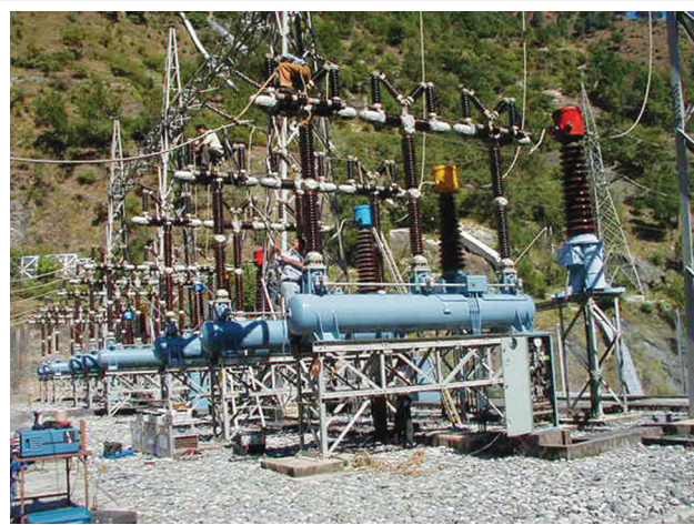
A VIEW OF CIRCUIT BREAKERS
