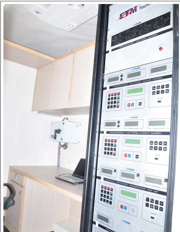
A VIEW OF CONTROL PANEL OF MOBILE FIELD CT/PT TESTING
