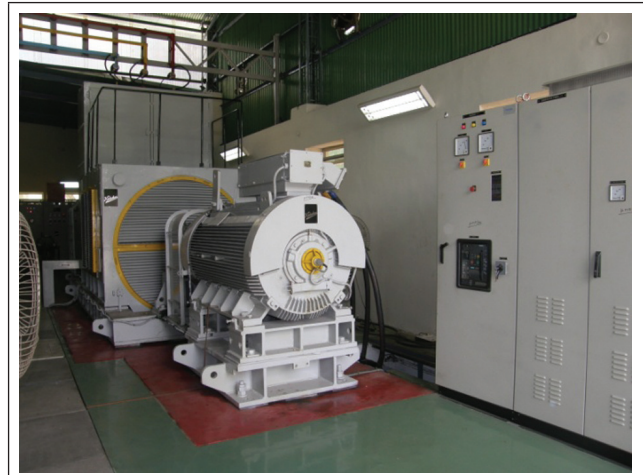
PHOTOGRAPH SHOWING THE NEW 50 MVA SC GENERATOR WITH DRIVE MOTOR AND VFD
