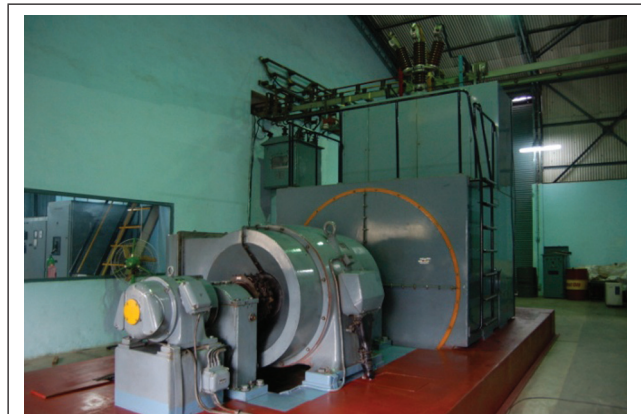
PHOTOGRAPH SHOWING THE OLD 50 MVA SC GENERATOR
