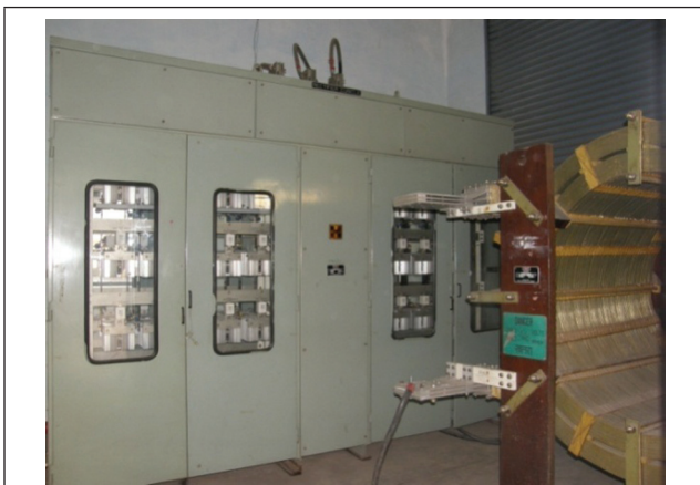
PHOTOGRAPH SHOWING THE DC TEST FACILITY
