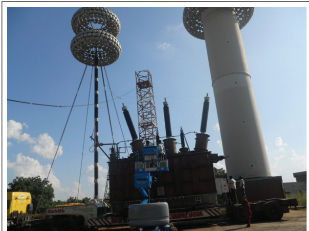
FIG. 35 100 MVA, 230/110/11 kV AUTO TRANSFORMER
