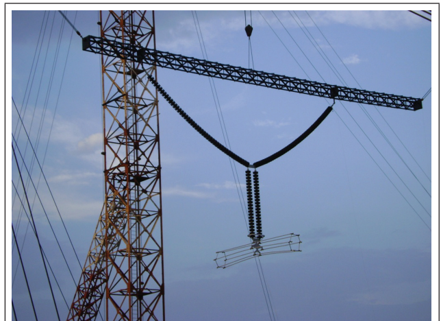
FIG. 32 800 kV DC - "Y" INSULATOR STRING
