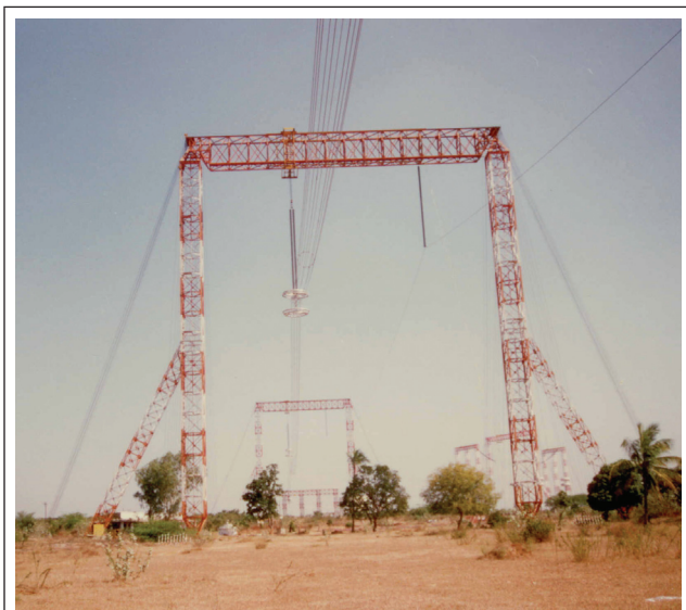
FIG. 15 A VIEW OF EXPERIMENTAL TRANSMISSION LINE
