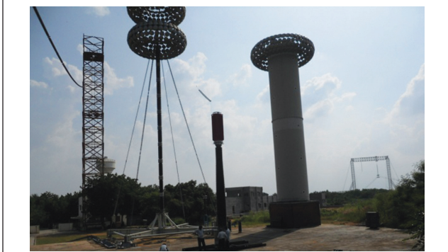
FIG. 29 765 kV CURRENT TRANSFORMERS
