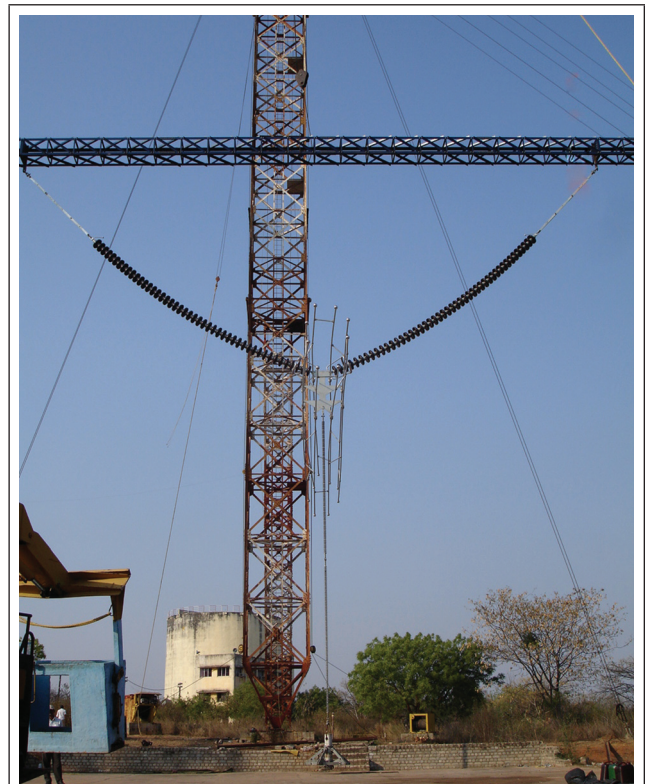
FIG. 21 A VIEW OF 1200 kV SINGLE 'V' SUSPENSION STRING
