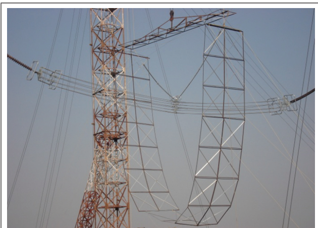
FIG. 6 TEST SET UP WITH BUNDLE CONDUCTOR ALONG WITH INSULATOR STRING AND TOWER WINDOW SIMULATION
