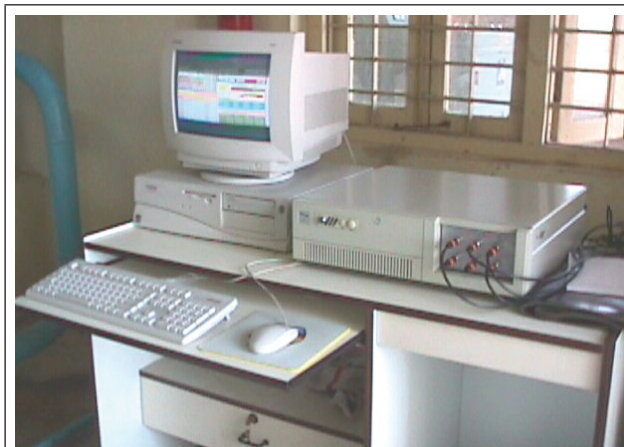
FIG. 25 DATA ACQUISITION SYSTEM FOR ON-LINE LEAKAGE CURRENT MEASUREMENT
