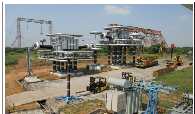
FIG. 14 A VIEW OF 1600 kV/6 A CASCADE TRANSFORMER
