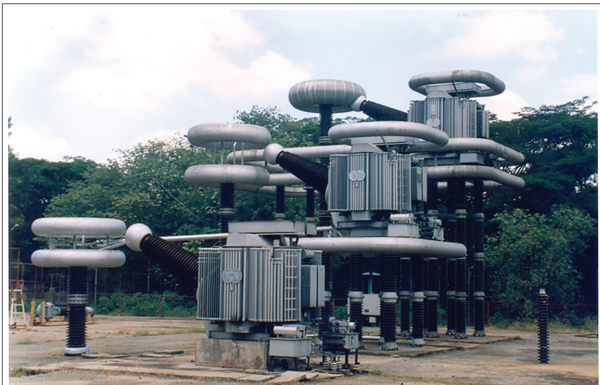
THE 1800 kV TUR MAKE POWER FREQUENCY TEST VOLTGE SOURCE (CASCADE TRANSFORMER)
