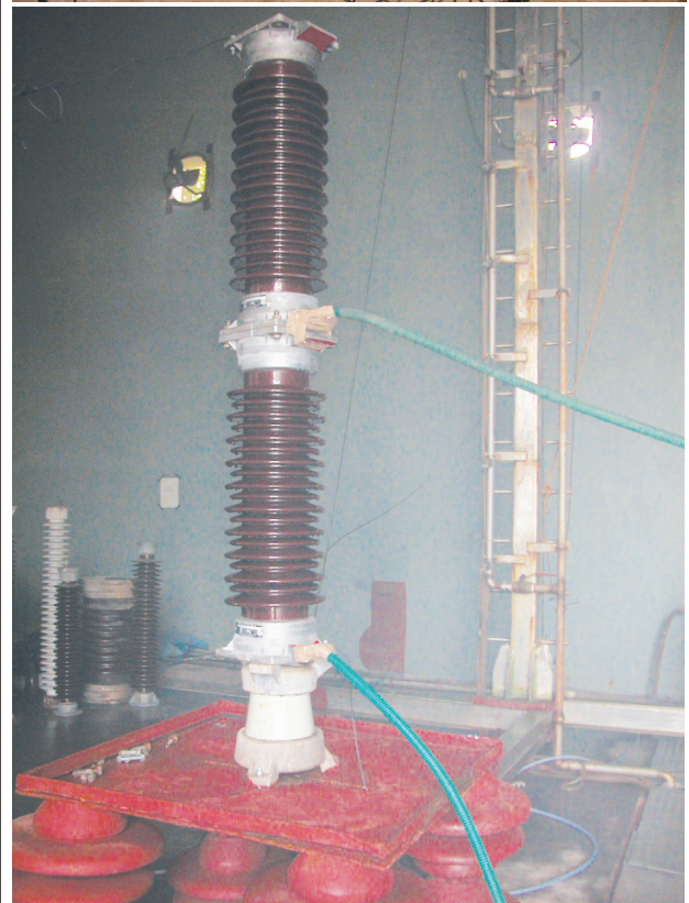
ARRANGEMENTS UNDER WAY FOR POLLUTION TEST ON ZINC OXIDE SURGE ARRESTER
