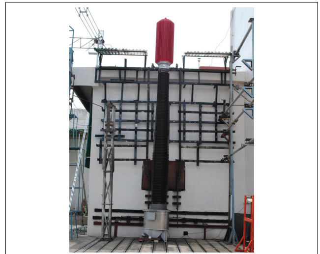
FIG. 18 800 kV CURRENT TRANSFORMER
