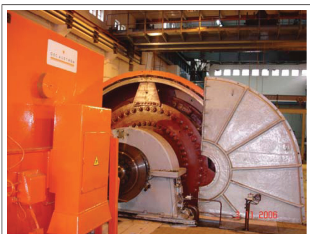
FIG. 9 ALSTOM MAKE 1500 MVA SC GENERATOR
