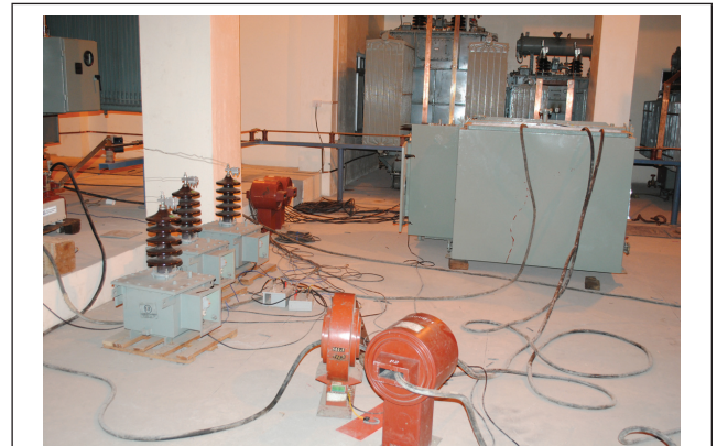
FIG. 19 OLTC UNDER TEST
