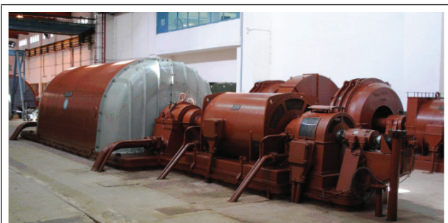
FIG. 1 OERLIKON MAKE 1500 MVA SC GENERATOR
