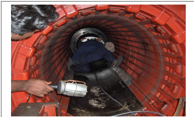
FIG. 21 SC GENERATOR STATOR
