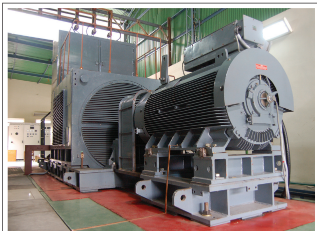
50 MVA SHORT CIRCUIT GENERATOR AT CPRI
