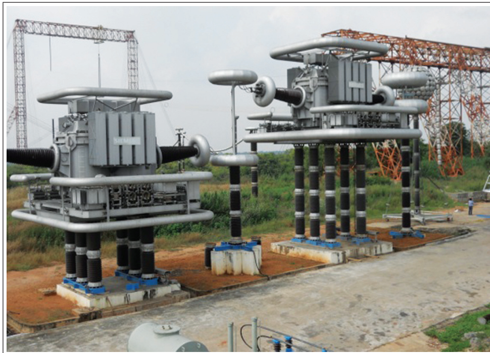
1600 kV, 9600 kVA CASCADED TRANSFORMER AT UHVRL, HYDERABAD
