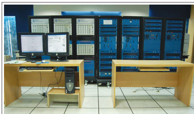
REAL-TIME DIGITAL SIMULATOR FACILITY
