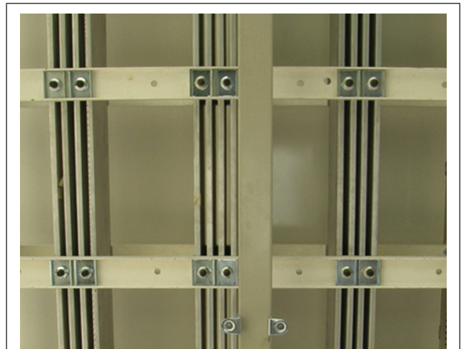
FIG. 7 SELF EXTINGUISHABLE FIBER MATERIAL BUS-BAR SUPPORT WITH MS CLAMPS.
