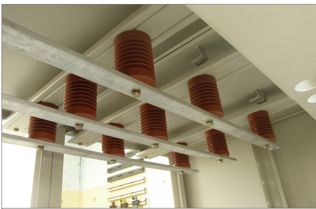
FIG. 3 EPOXY RESIN CAST BUS-BAR SUPPORT.
