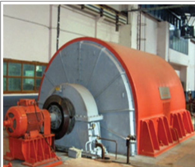
FIG. 3 ACTUAL VIEW OF 1900 MVA SHORT CIRCUIT GENERATOR
