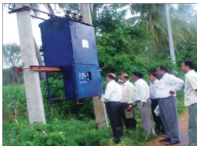
FIG. 1 VERIFICATION OF FEEDER METER
