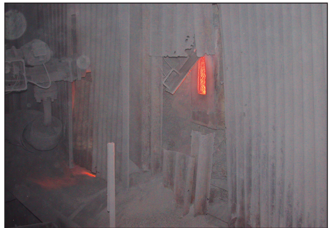
DAMAGED INSULATION AND HEAT LEAK FROM FURNACE-2
