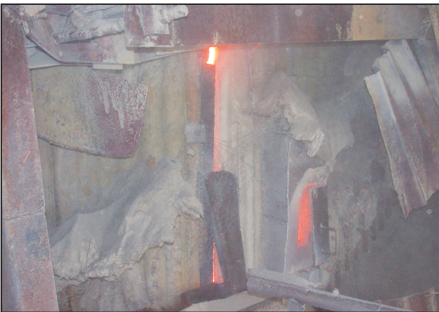
DAMAGED INSULATION AND HEAT LEAK FROM FURNACE-1
