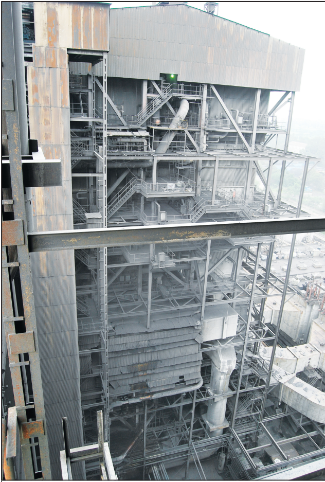
VIEW OF BOILER-3
