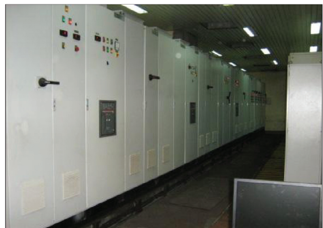
FIG. 6 NEW DRIVES PANEL WITH CENTER FEED CONVERTER RRU
