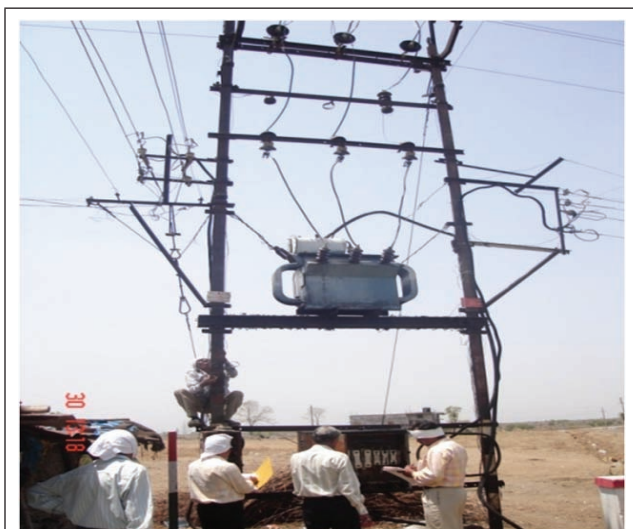
FIG. 7 11 KV DTC DURING INSPECTION
