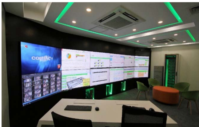
Figure 2. Smart, connected devices are the first step in a completely digitized power distribution system.
