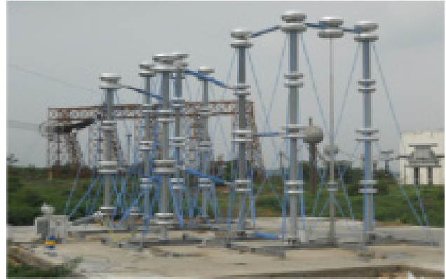
Figure 1. \pm 1200 kV HVDC source.
