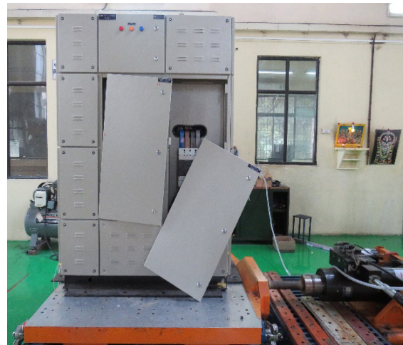
Figure 8. Panel door dislocated.
