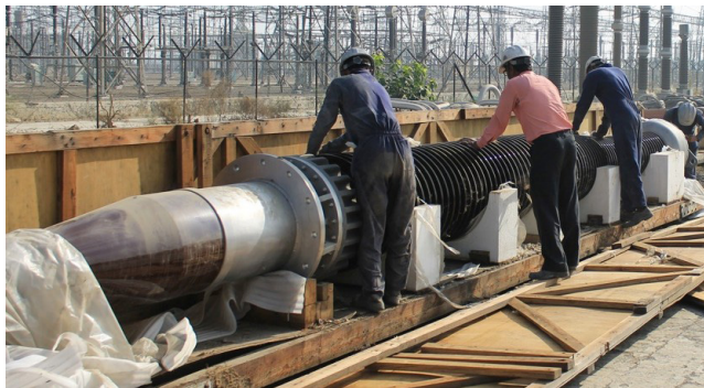
Figure 3. Unpacking the bushing.
